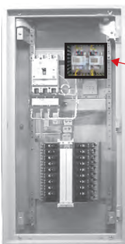
Example of installation inside board
