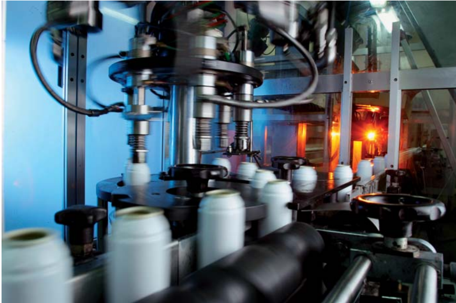
Can filling plant controlled by Mitsubishi GOTs
